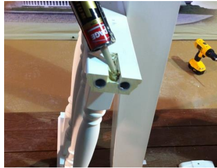
20. Apply a ½" bead of a urethane based construction adhesive to the underside of each end of the top and bottom rail, where the angle brackets will meet.
